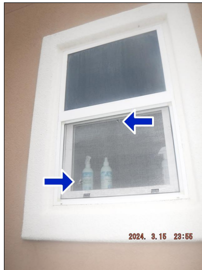
1.2 Item 2(Picture) Damage screen (back of home)
