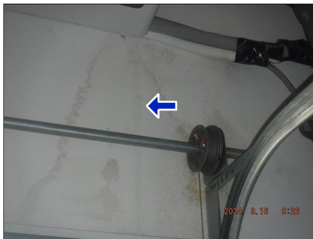
5.1 Item 2(Picture) Moisture stains
