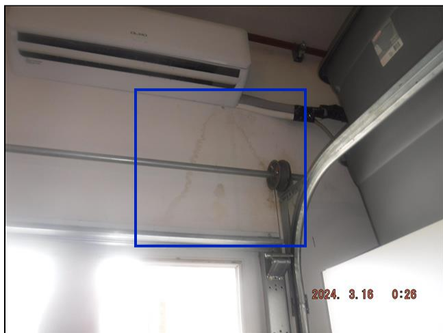
5.1 Item 1(Picture) Wall stains under a/c unit
