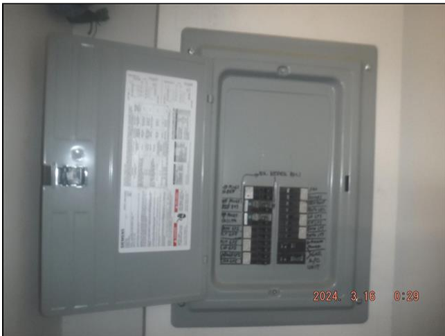
2.3 Item 3(Picture) Sub Electrical Panel
