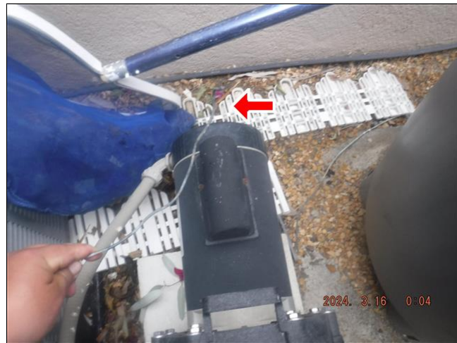
11.5 Item 2(Picture) Pump not grounded
