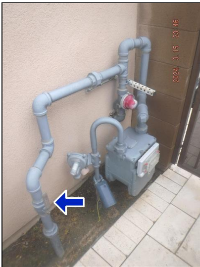
3.7 Item 2(Picture) Pool heater gas valve
