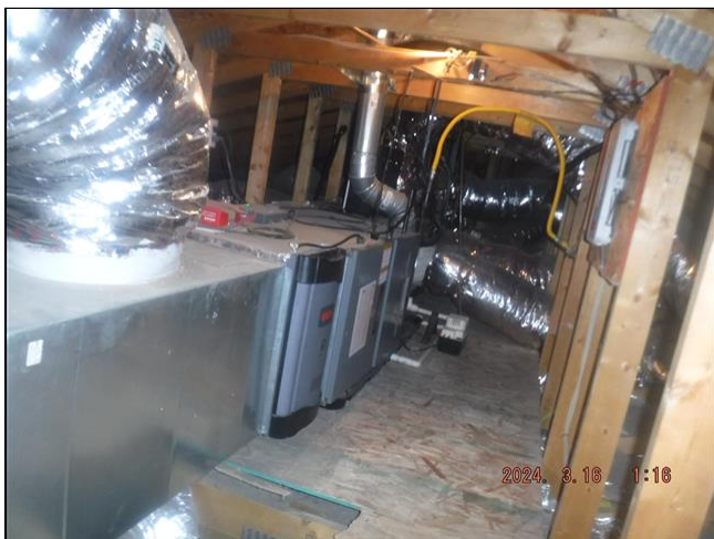
4.0 Item 1(Picture) Air Heating Unit
