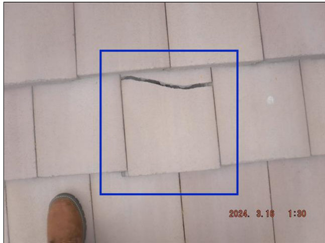
10.0 Item 4(Picture) Cracked/damage tile
