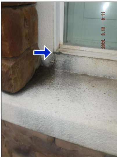
1.2 Item 5(Picture) Stained sill
