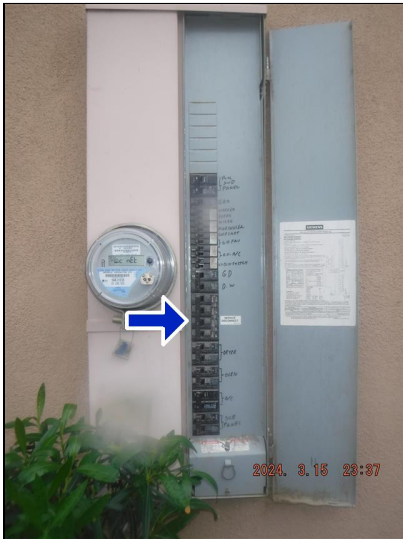
2.3 Item 1(Picture) Main electrical shut off (at panel)
