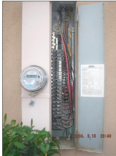
2.3 Item 2(Picture) Electrical Wiring/Conductors
