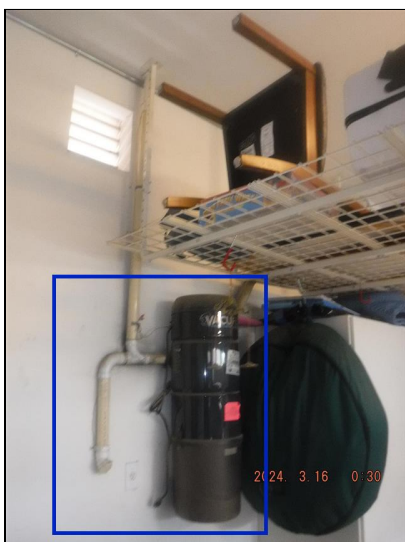
3.16 Item 1(Picture) Central vacuum system
