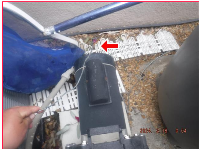
11.5 Item 2(Picture) Pump not grounded
