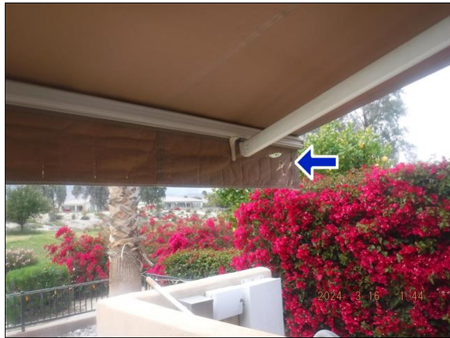
10.5 Item 4(Picture) Torn flaps
