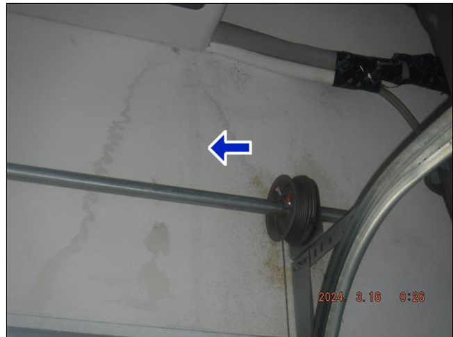
5.1 Item 2(Picture) Moisture stains
