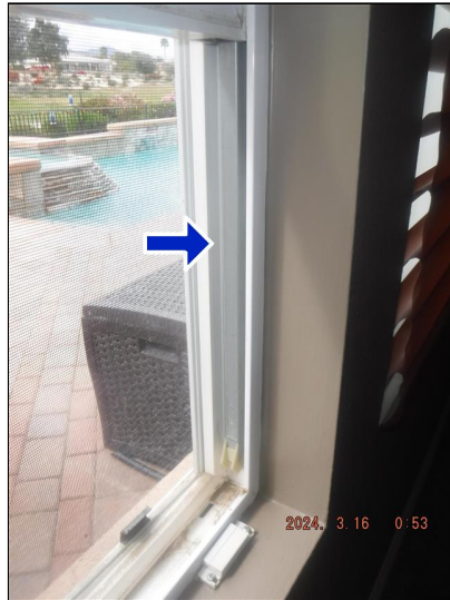
6.5 Item 2(Picture) Window spring loose
