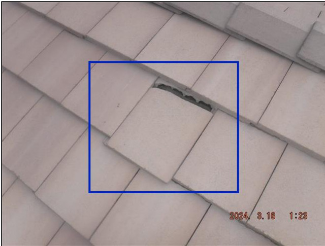
10.0 Item 1(Picture) Cracked/damage tile
