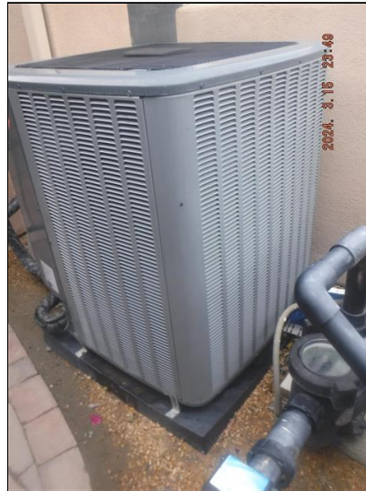
4.5 Item 2(Picture) Air Cooling Unit
