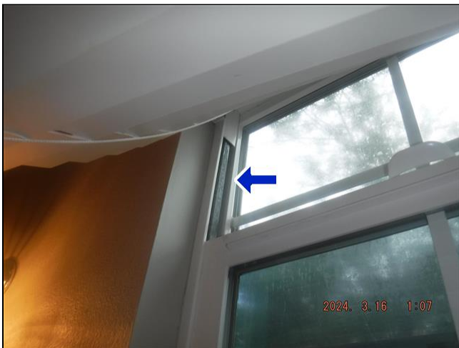
6.5 Item 4(Picture) Window spring loose
