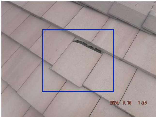
10.0 Item 1(Picture) Cracked/damage tile
