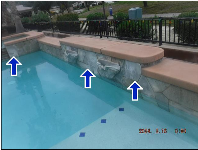
11.1 Item 1(Picture) Calcium build up on walls
