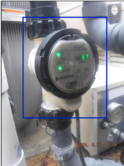
11.3 Item 1(Picture) Pool chlorine generator unit
