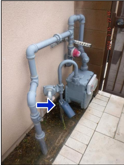
3.7 Item 1(Picture) Main Gas Shut Off (At Meter)
