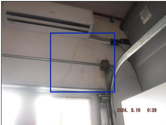
5.1 Item 1(Picture) Wall stains under a/c unit
