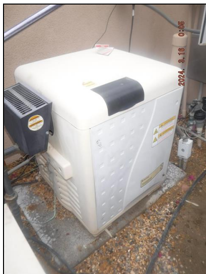
11.8 Item 1(Picture) Pool heating unit
