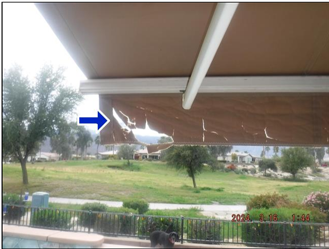
10.5 Item 3(Picture) Torn flaps
