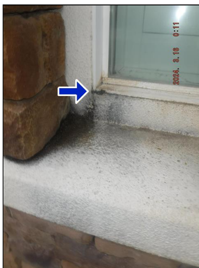
1.2 Item 5(Picture) Stained sill
