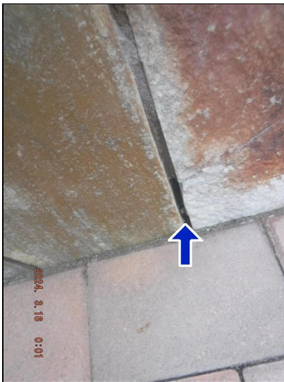
11.2 Item 1(Picture) Tile mortar failing
