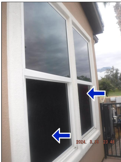
1.2 Item 1(Picture) Missing screens (right side of home)
