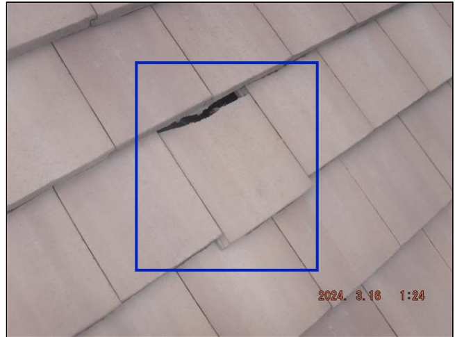
10.0 Item 2(Picture) Cracked/damage tile
