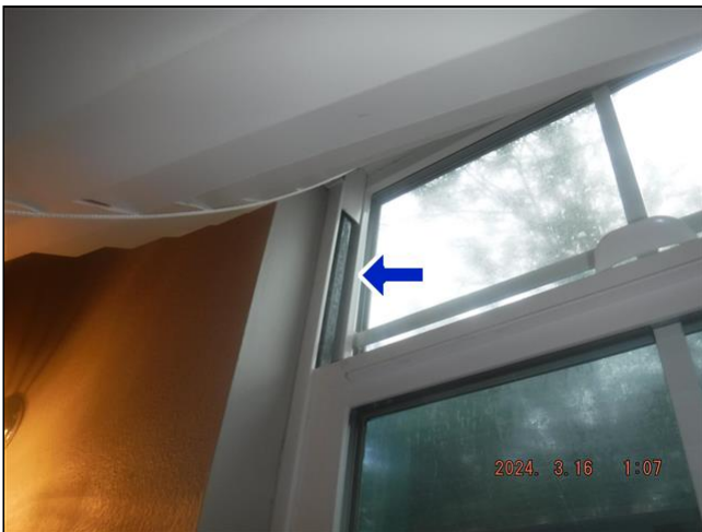
6.5 Item 4(Picture) Window spring loose
