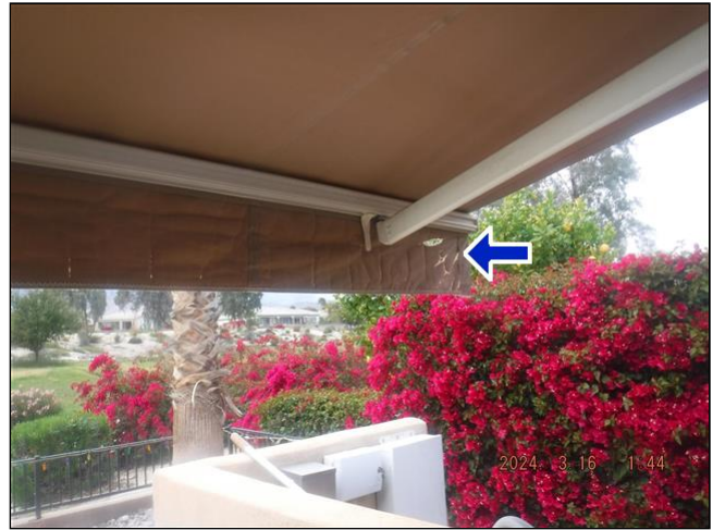
10.5 Item 4(Picture) Torn flaps
