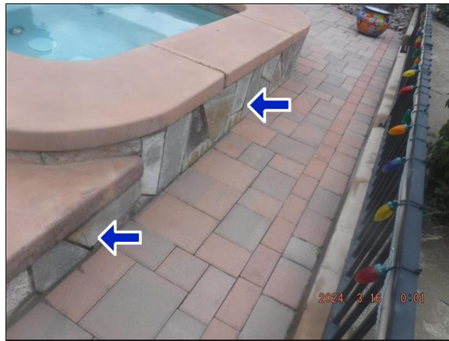
11.2 Item 2(Picture) Tile mortar failing
