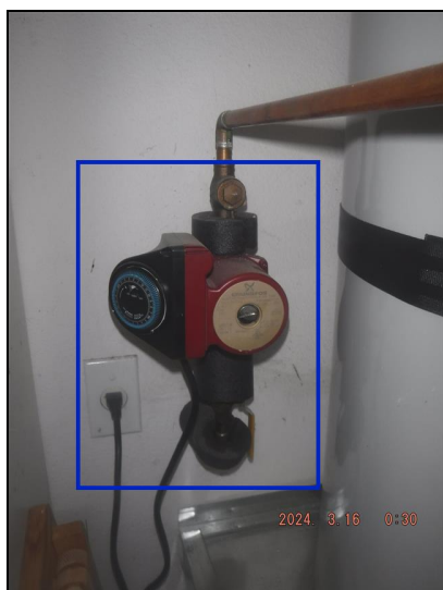
3.5 Item 1(Picture) Recirculating pump
