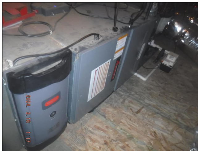
4.0 Item 2(Picture) Air Heating Unit
