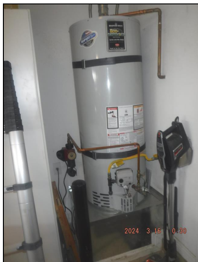
3.4 Item 1(Picture) Water Heater Unit
