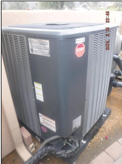
4.5 Item 1(Picture) Air Cooling Unit
