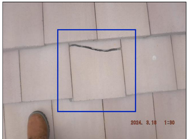
10.0 Item 4(Picture) Cracked/damage tile
