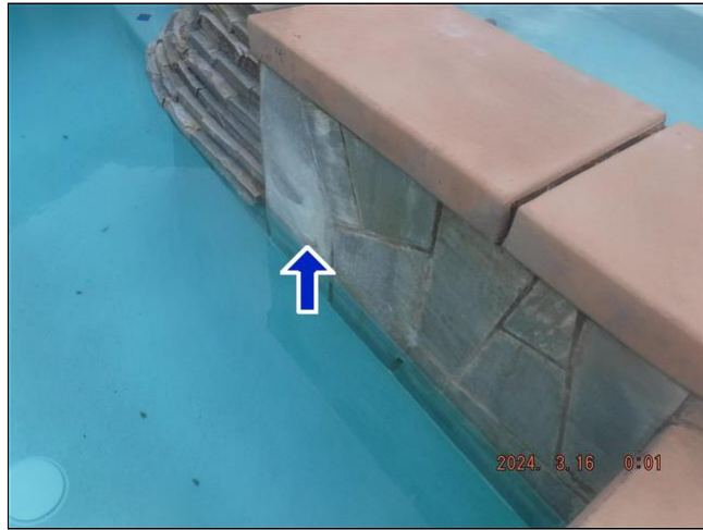
11.1 Item 2(Picture) Calcium build up on walls
