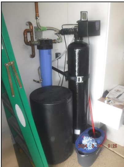
3.12 Item 1(Picture) water softener/filtration system
