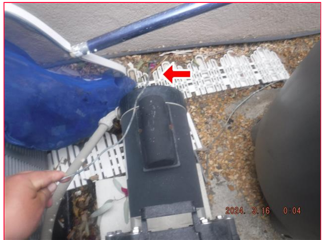
11.5 Item 2(Picture) Pump not grounded
