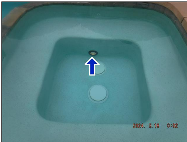
11.11 Item 2(Picture) Spa light
