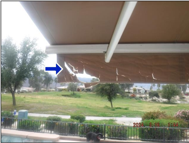
10.5 Item 3(Picture) Torn flaps
