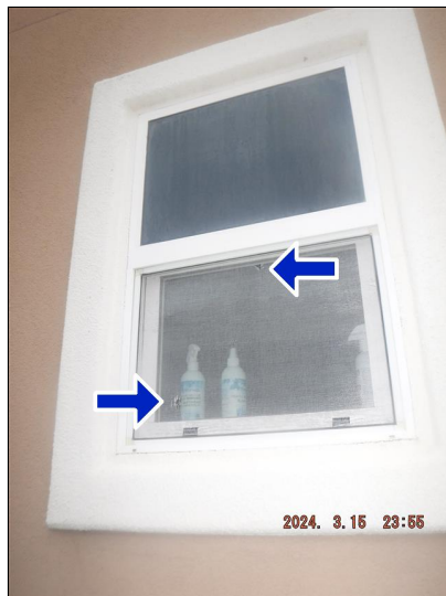
1.2 Item 2(Picture) Damage screen (back of home)
