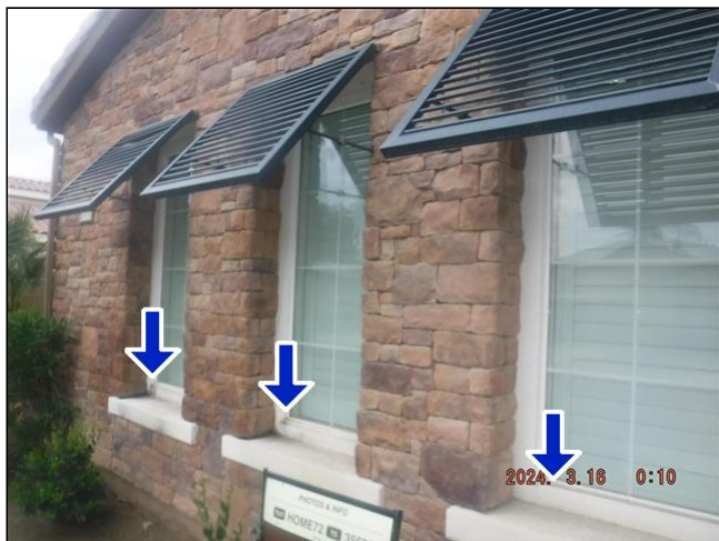
1.2 Item 3(Picture) Windows front of home
