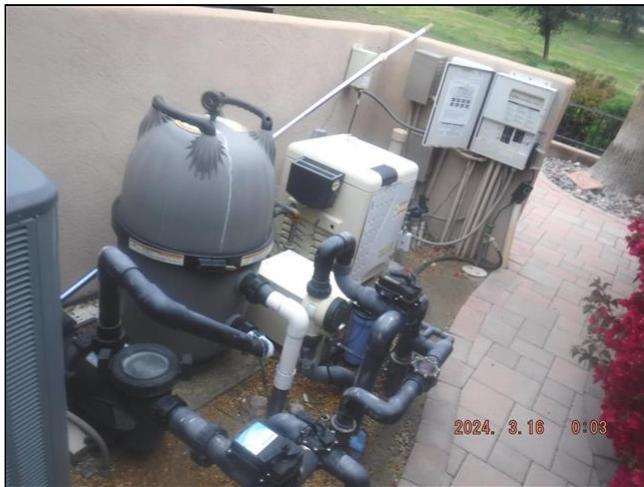
POOL FILTRATION SYSTEM
