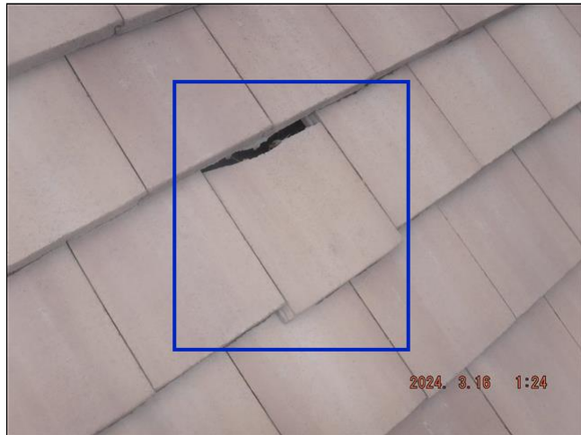
10.0 Item 2(Picture) Cracked/damage tile
