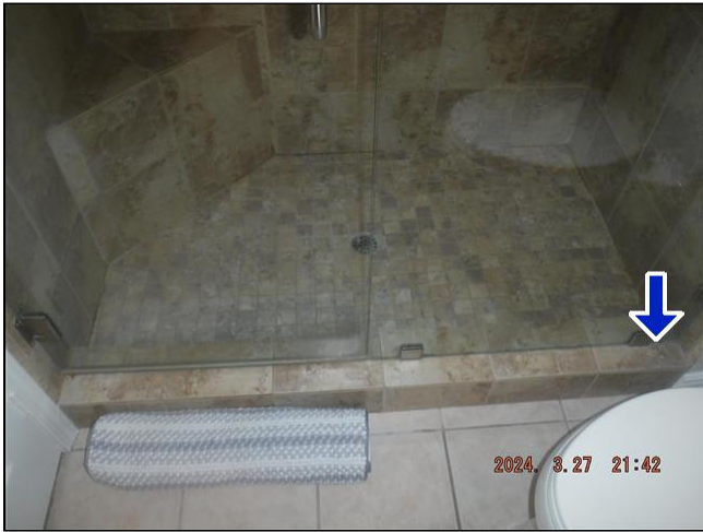
3.11 Item 1(Picture) Location of shower stall leak
