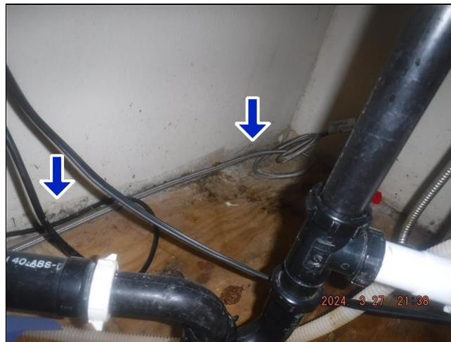
6.1 Item 4(Picture) Black substance on wall
