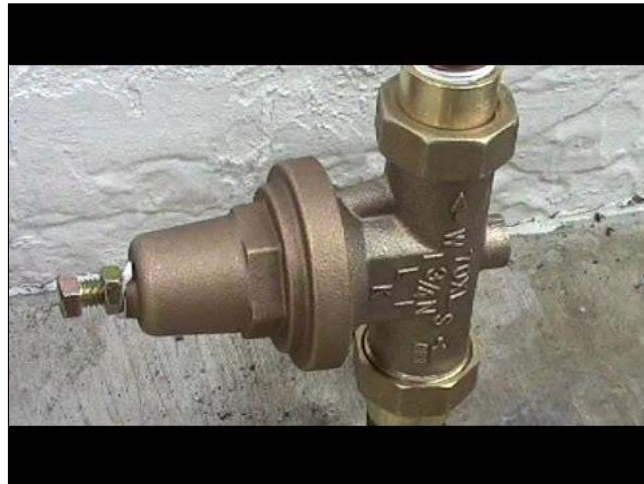
3.5 Item 2(Picture) Example of a water pressure regulator
