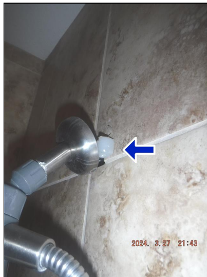
3.10 Item 2(Picture) Loose shower head
