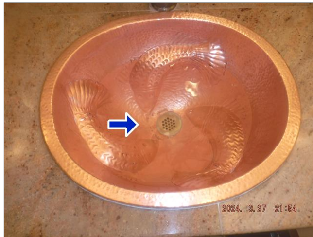
3.0 Item 2(Picture) Sink drains slow
