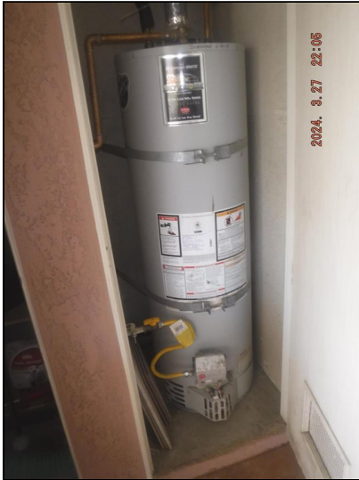
3.6 Item 1(Picture) Water Heater Unit
