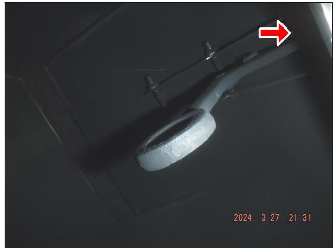
4.6 Item 2(Picture) Fireplace damper
