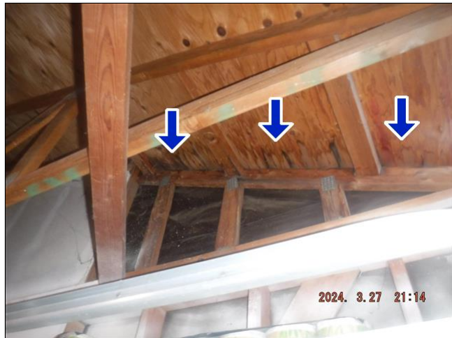
5.0 Item 2(Picture) Stained plywood sheathing
