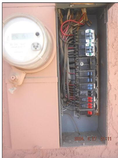
2.3 Item 2(Picture) Electrical Wiring/Conductors
