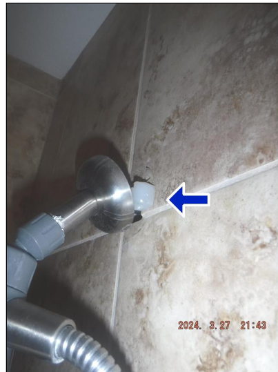
3.10 Item 2(Picture) Loose shower head
