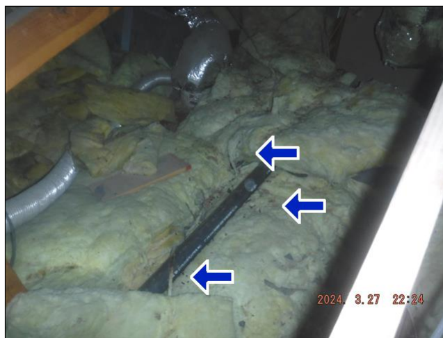
8.4 Item 2(Picture) Rodent droppings
