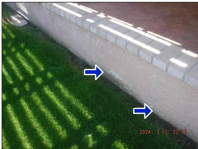
1.4 Item 3(Picture) Stucco coating peeling
