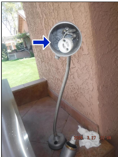
2.6 Item 1(Picture) BBQ light fixture
