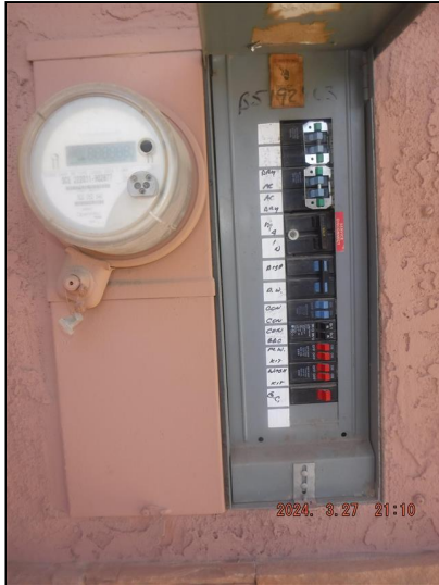
2.1 Item 1(Picture) No AFCI breakers in panel
