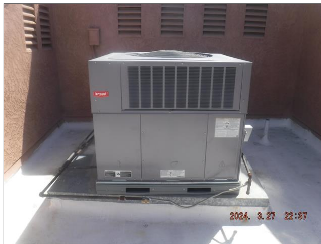
4.7 Item 2(Picture) Air Cooling Unit
