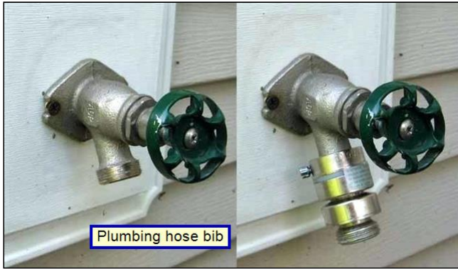
3.3 Item 3(Picture) Example of hose bib with a anti-siphon valve
