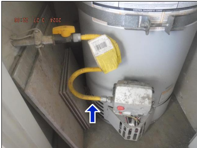
3.7 Item 1(Picture) Water heater gas line
