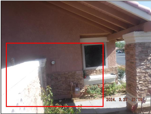
3.8 Item 2(Picture) Location of gas odor detected
