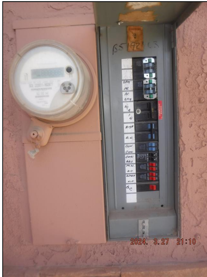
2.1 Item 1(Picture) No AFCI breakers in panel
