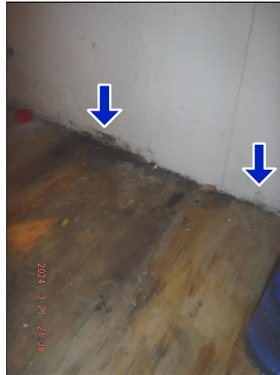
6.1 Item 2(Picture) Black substance on wall
