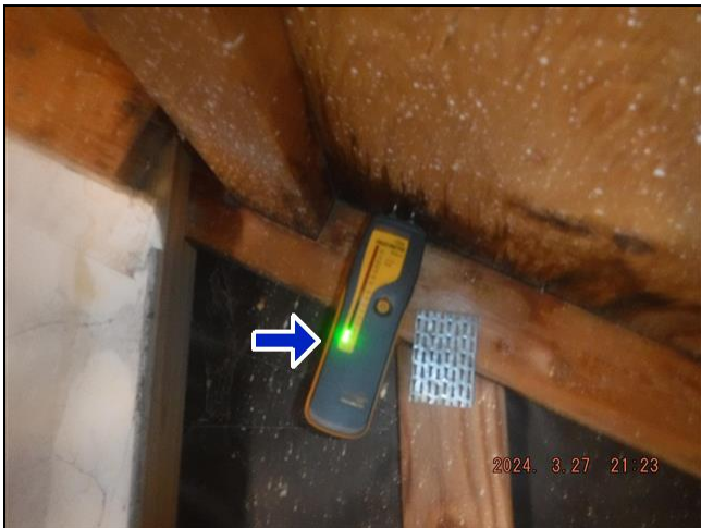
5.0 Item 3(Picture) Moisture meter (device) indicated dry surface
