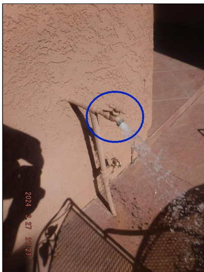
3.3 Item 1(Picture) Plumbing hose bib (front of home)
