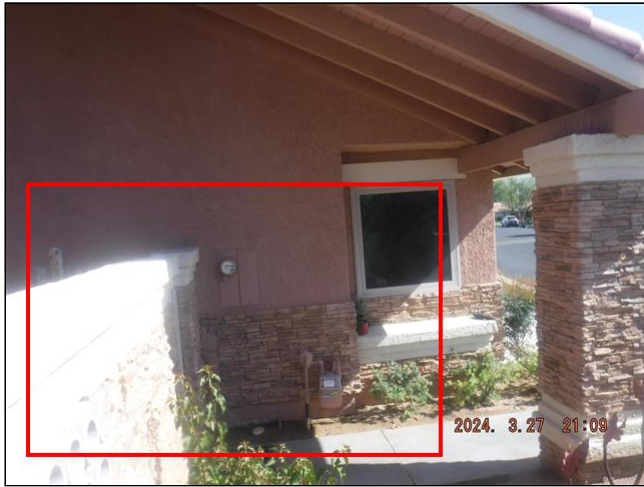
3.8 Item 2(Picture) Location of gas odor detected
