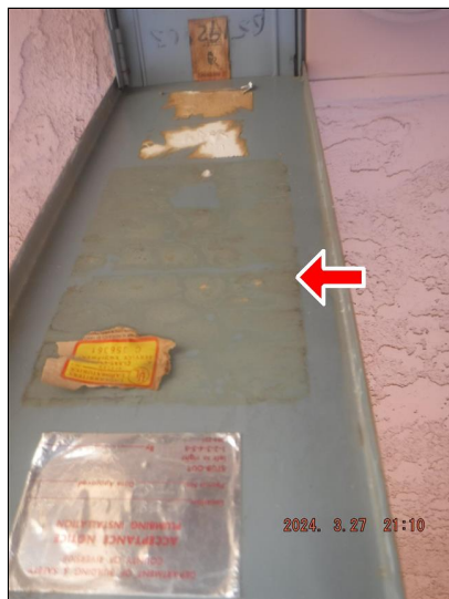
2.1 Item 2(Picture) Missing panel label
