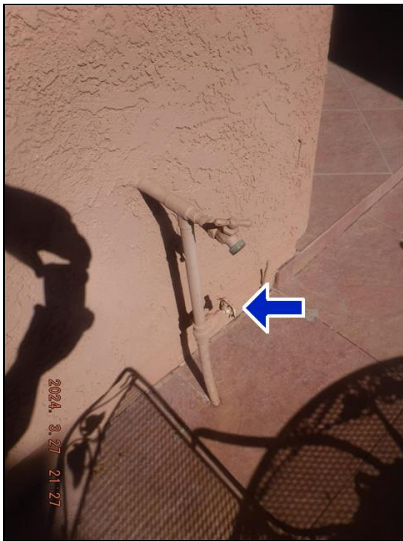
3.2 Item 2(Picture) Water shut off valve
