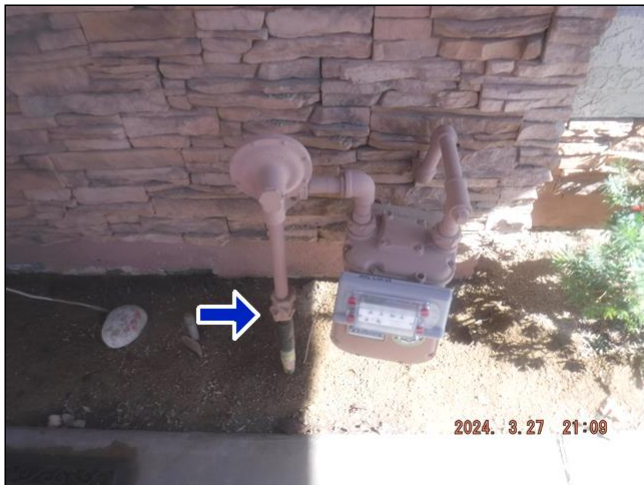
3.8 Item 1(Picture) Main Gas Shut Off (At Meter)
