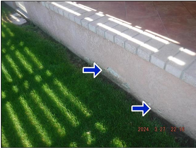
1.4 Item 3(Picture) Stucco coating peeling
