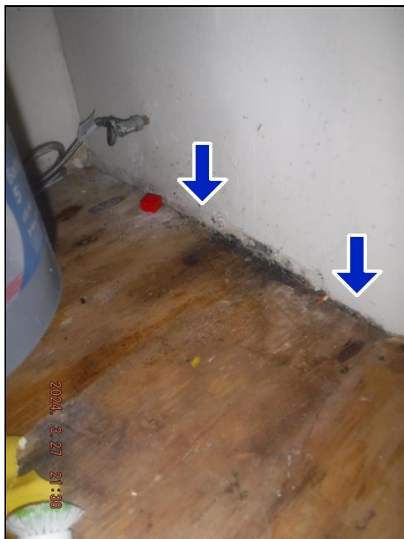
6.1 Item 3(Picture) Black substance on wall
