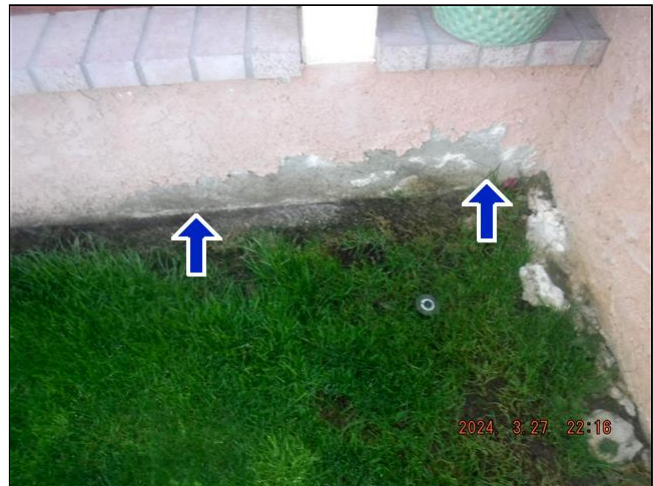
1.4 Item 2(Picture) Stucco coating peeled off
