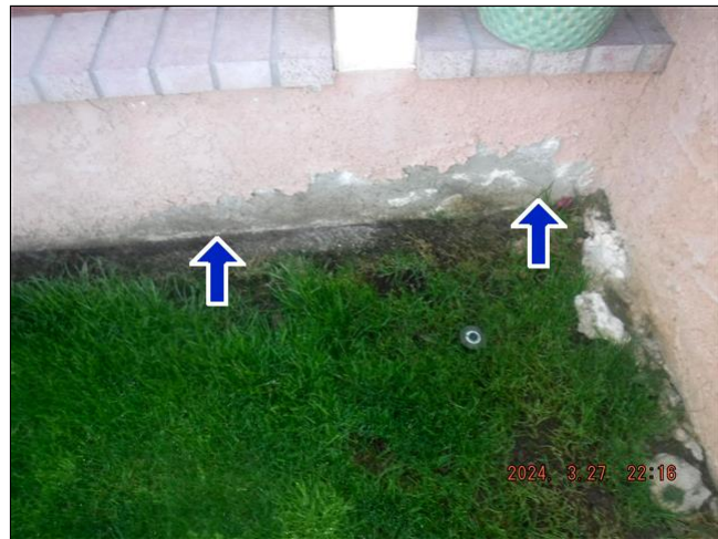
1.4 Item 2(Picture) Stucco coating peeled off
