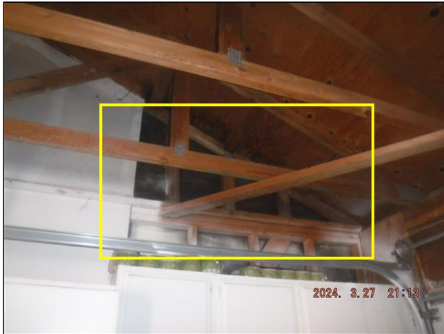
5.0 Item 1(Picture) Location of ceiling water stains
