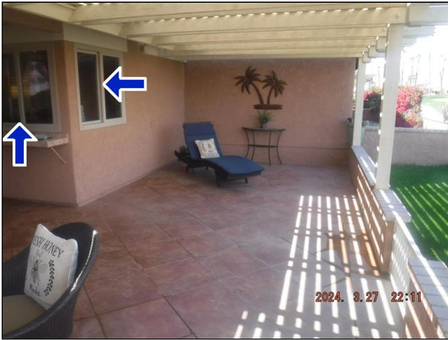
1.2 Item 1(Picture) Windows missing screens
