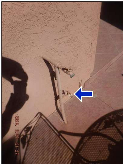
3.2 Item 2(Picture) Water shut off valve
