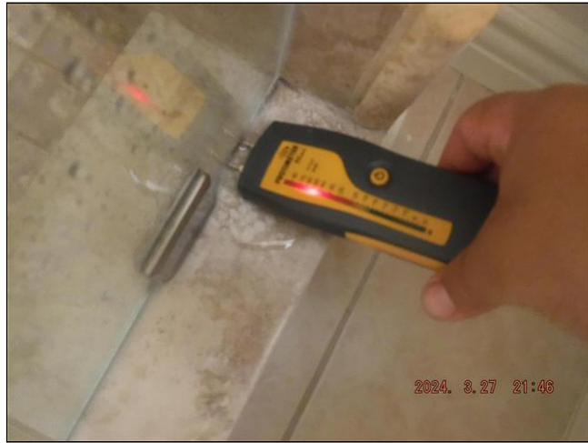
3.11 Item 2(Picture) Shower stall leak
