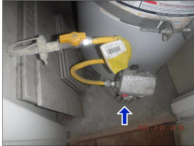
3.6 Item 2(Picture) No drain pan
