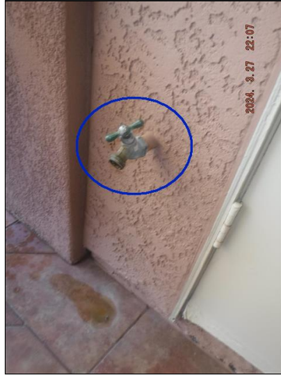
3.3 Item 2(Picture) Plumbing hose bib (patio)
