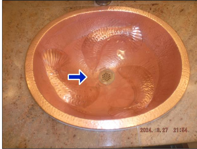
3.0 Item 2(Picture) Sink drains slow
