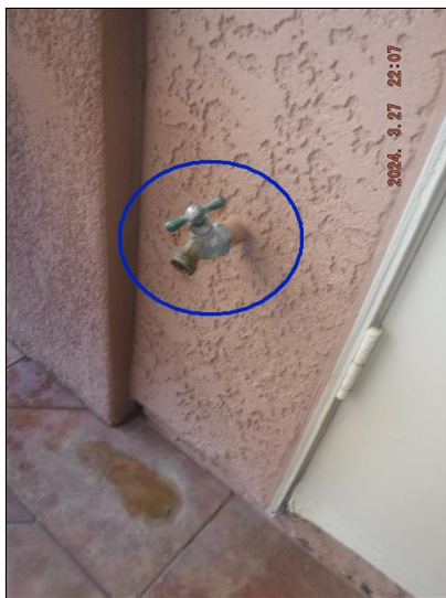
3.3 Item 2(Picture) Plumbing hose bib (patio)
