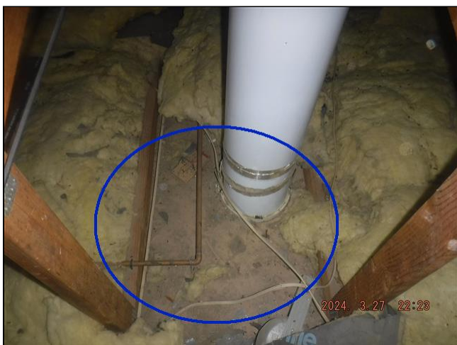
8.4 Item 1(Picture) Rodent droppings
