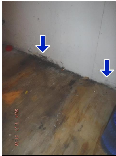
6.1 Item 2(Picture) Black substance on wall
