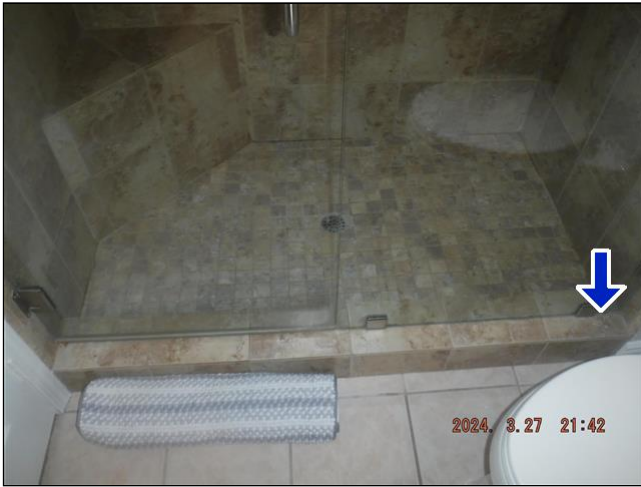
3.11 Item 1(Picture) Location of shower stall leak
