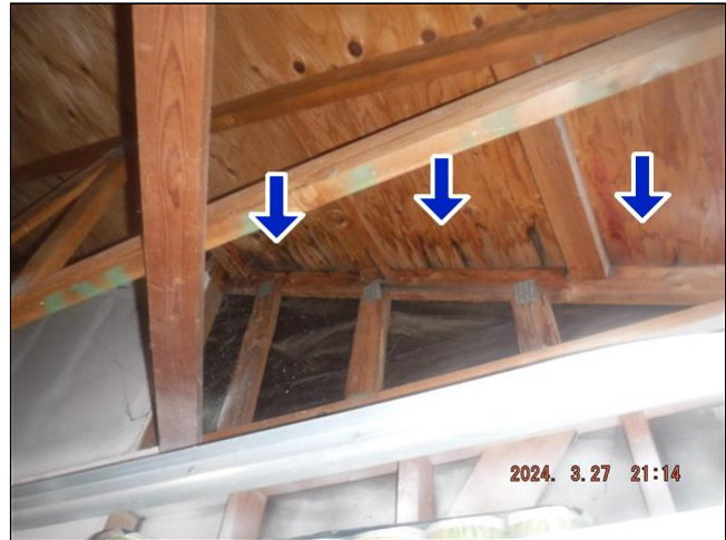
5.0 Item 2(Picture) Stained plywood sheathing
