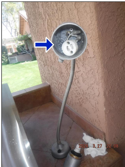
2.6 Item 1(Picture) BBQ light fixture
