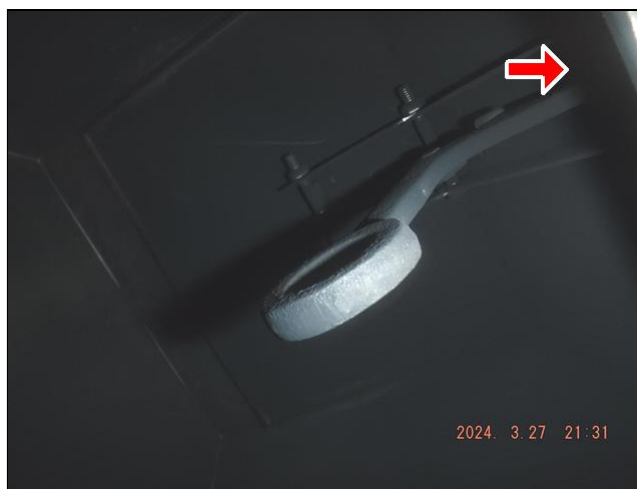
4.6 Item 2(Picture) Fireplace damper
