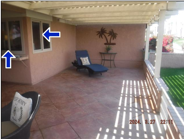
1.2 Item 1(Picture) Windows missing screens
