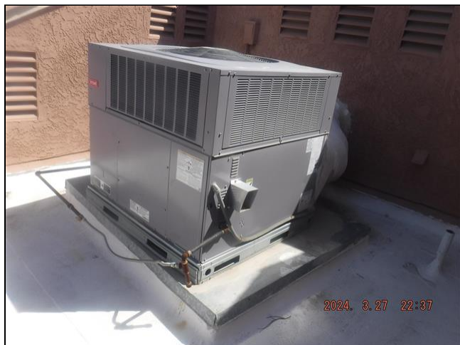
4.7 Item 1(Picture) Air Cooling Unit
