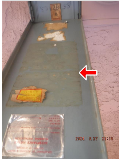
2.1 Item 2(Picture) Missing panel label
