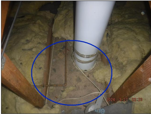
8.4 Item 1(Picture) Rodent droppings
