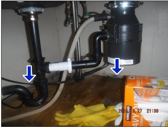
6.1 Item 1(Picture) Location of black substance
