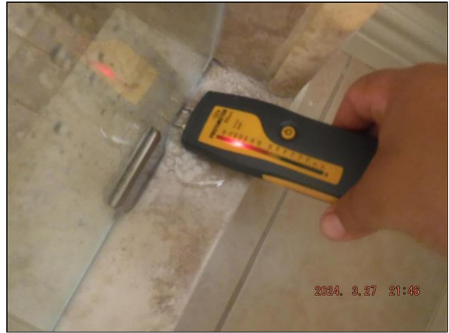
3.11 Item 2(Picture) Shower stall leak
