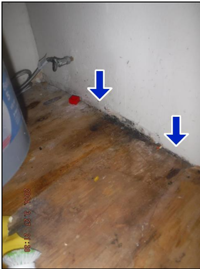
6.1 Item 3(Picture) Black substance on wall
