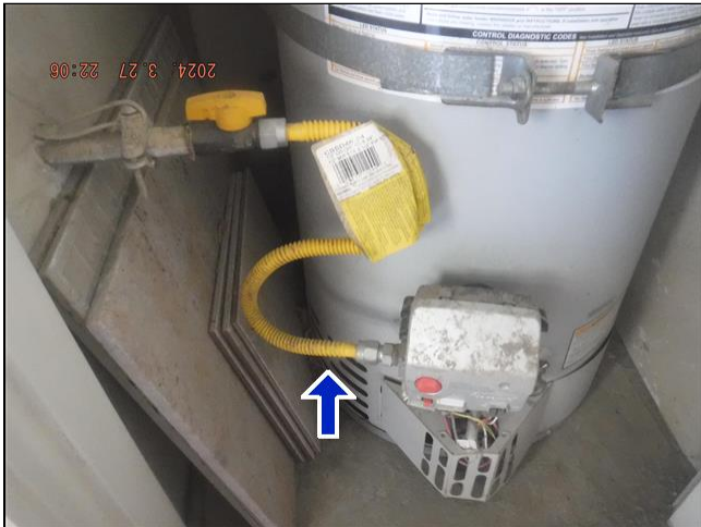
3.7 Item 1(Picture) Water heater gas line
