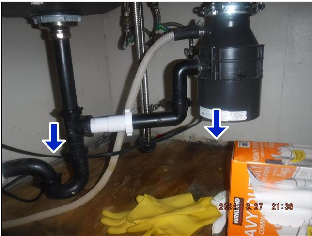
6.1 Item 1(Picture) Location of black substance
