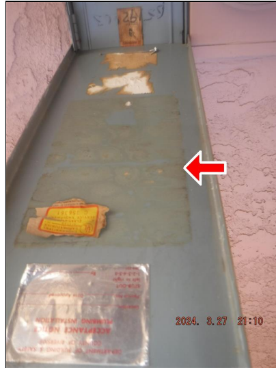
2.1 Item 2(Picture) Missing panel label
