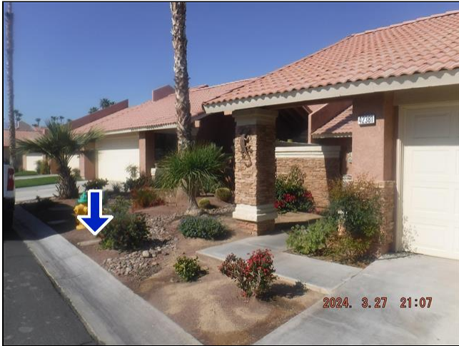
3.2 Item 1(Picture) Main Water Shut Off Valve and Meter
