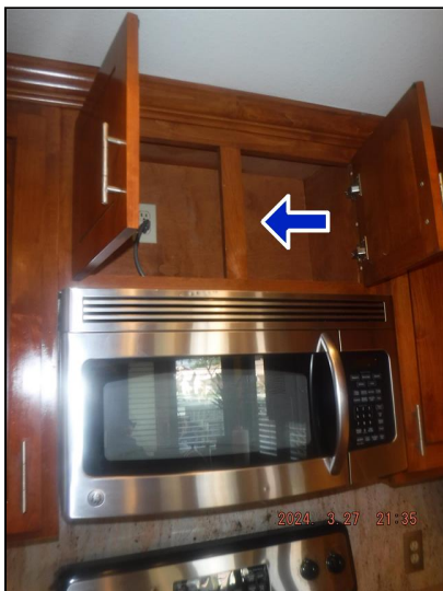
7.4 Item 1(Picture) No vent pipe for exhaust fan
