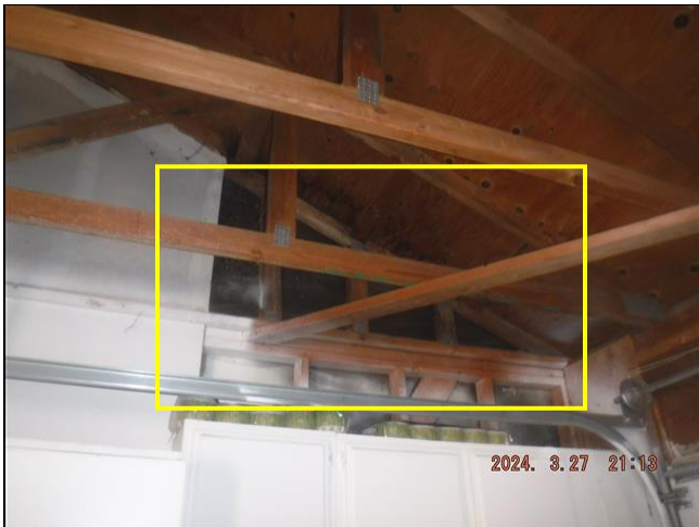
5.0 Item 1(Picture) Location of ceiling water stains
