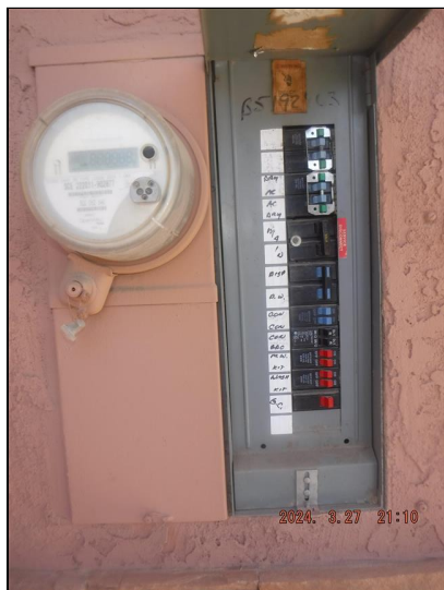
2.1 Item 1(Picture) No AFCI breakers in panel
