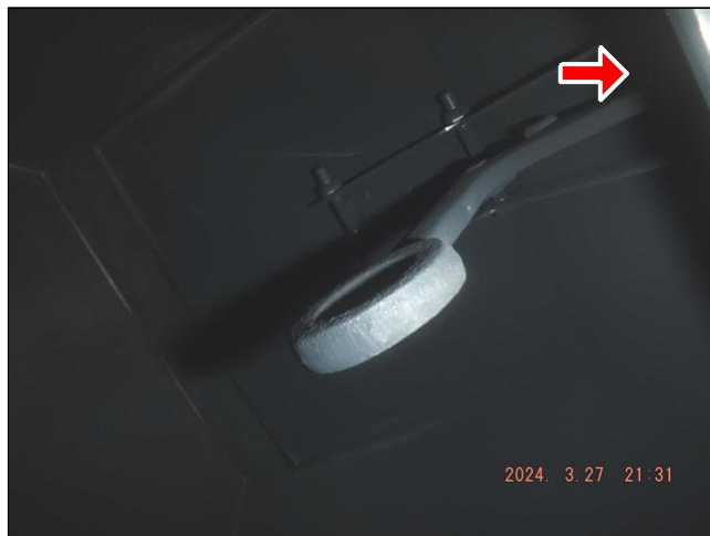
4.6 Item 2(Picture) Fireplace damper
