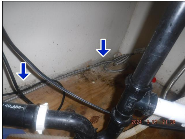
6.1 Item 4(Picture) Black substance on wall
