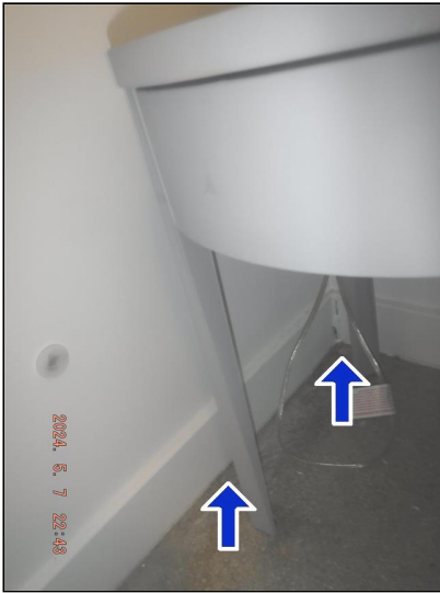
5.2 Item 3(Picture) Baseboard caulking failing
