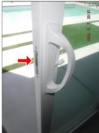
5.4 Item 4(Picture) Door did not lock properly
