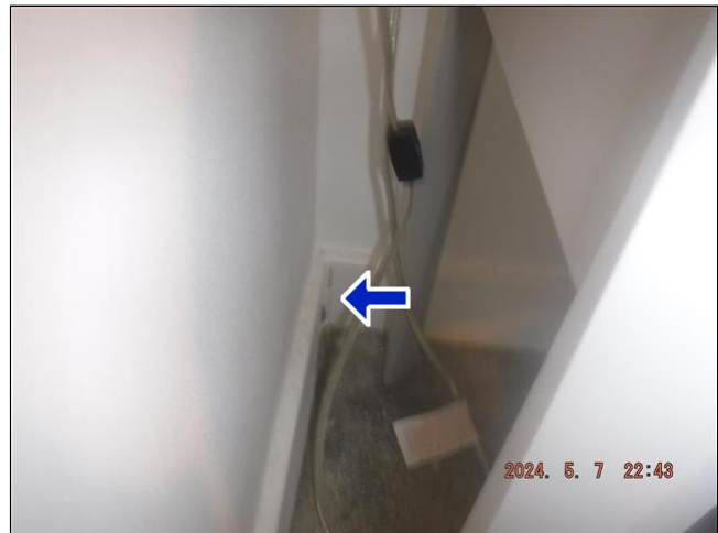
5.2 Item 2(Picture) Baseboard caulking failing
