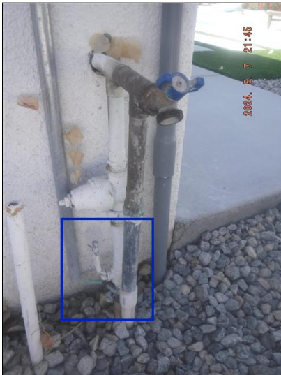
3.2 Item 1(Picture) Quick access water shut off valve location
