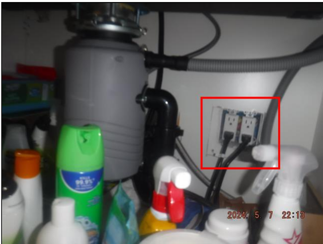
2.6 Item 5(Picture) Electrical outlet under kitchen sink
