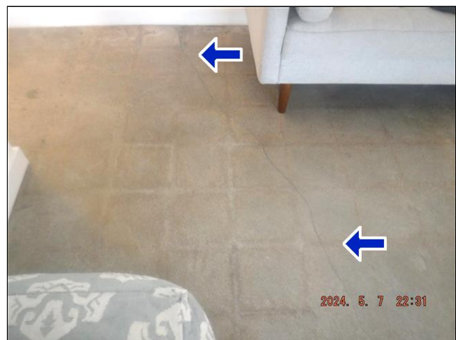
7.0 Item 2(Picture) Slab crack (living room)
