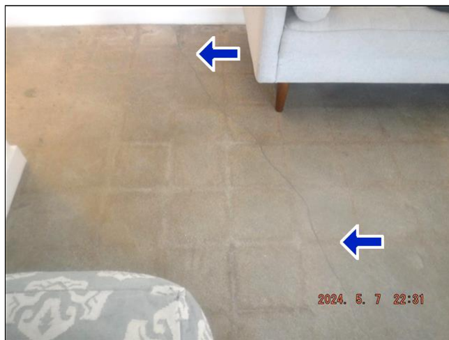
7.0 Item 2(Picture) Slab crack (living room)
