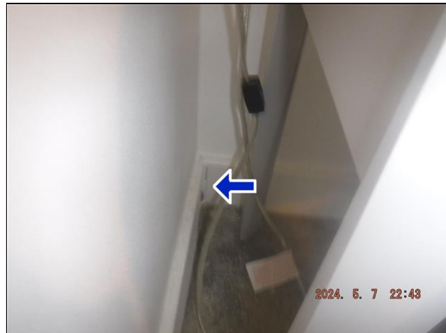
5.2 Item 2(Picture) Baseboard caulking failing
