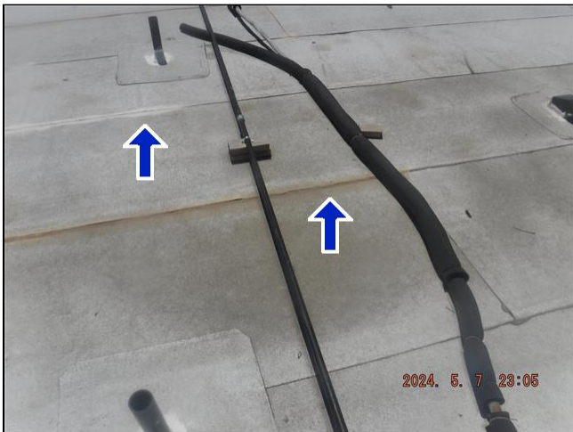
9.0 Item 3(Picture) Seem sealant failing
