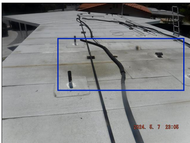
9.0 Item 5(Picture) Water ponding signs on roof
