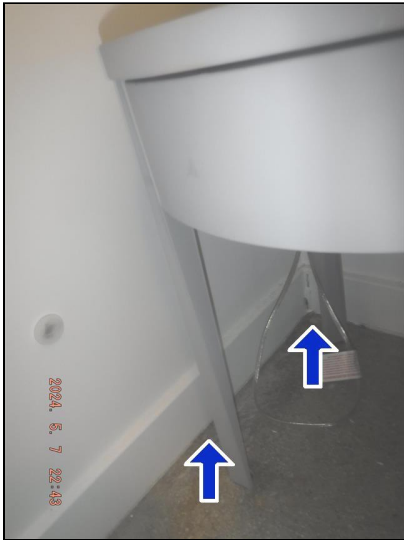
5.2 Item 3(Picture) Baseboard caulking failing
