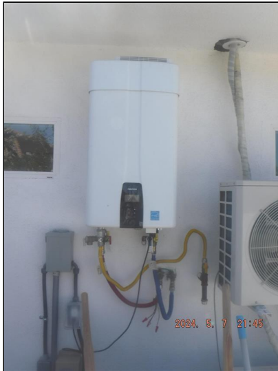
3.6 Item 1(Picture) Water Heater Unit
