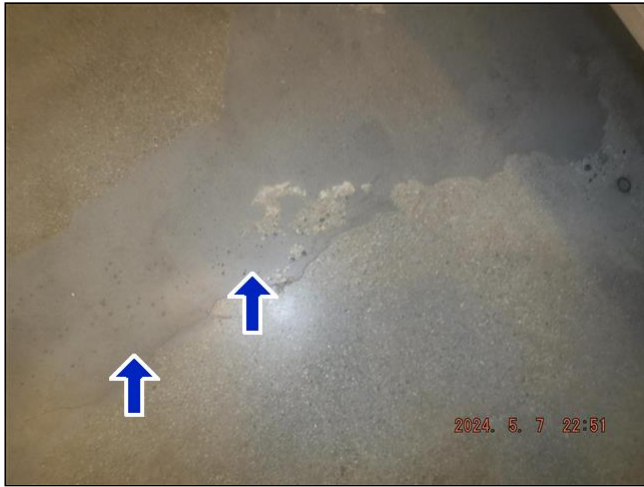
7.0 Item 3(Picture) Slab crack (master bath)
