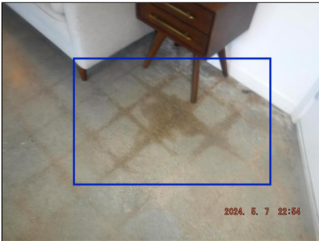
5.2 Item 5(Picture) Stained slab floor (living room)
