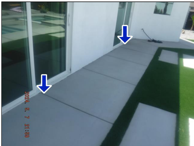
1.4 Item 3(Picture) Walkway slop, or near to door threshold
