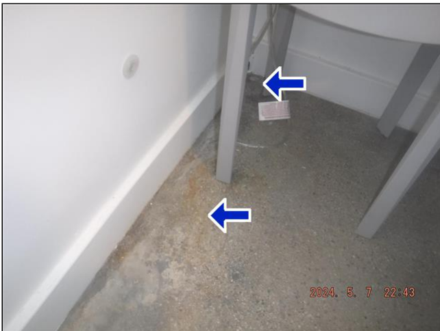
5.2 Item 1(Picture) Stained slab floor (guest bedroom)
