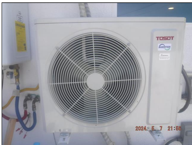
4.0 Item 3(Picture) Mini air conditioning unit 3
