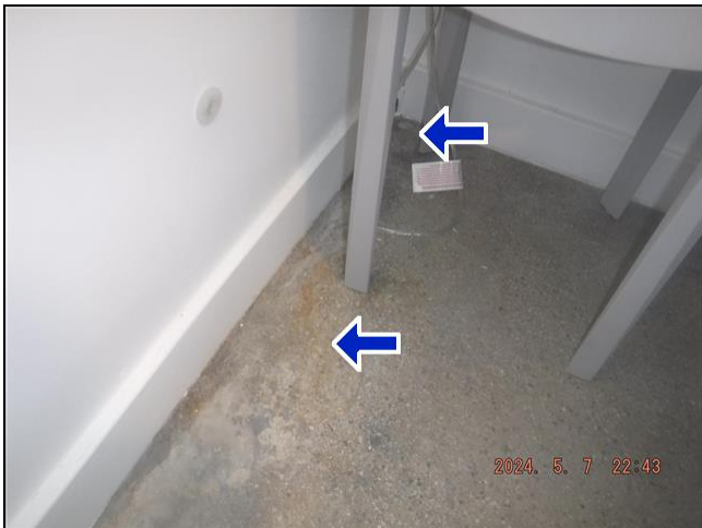
5.2 Item 1(Picture) Stained slab floor (guest bedroom)
