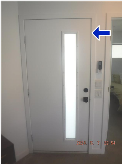
5.4 Item 1(Picture) Main entry door
