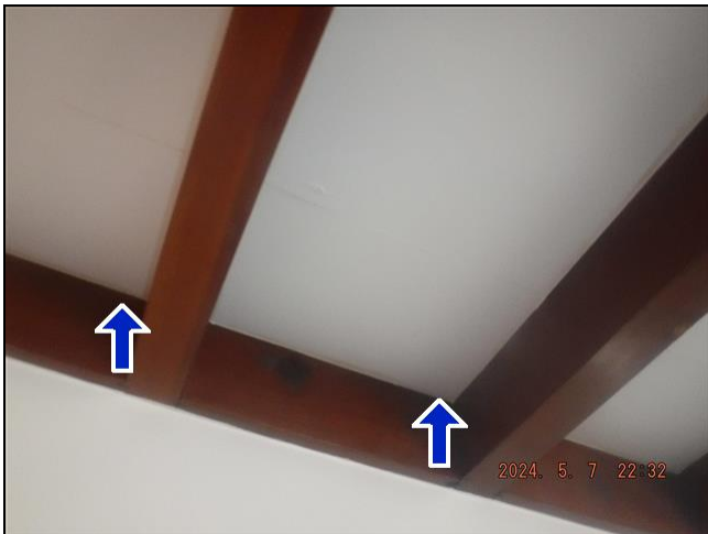
5.0 Item 3(Picture) Ceiling stains
