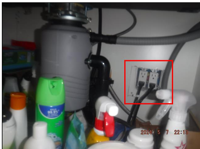
2.6 Item 5(Picture) Electrical outlet under kitchen sink
