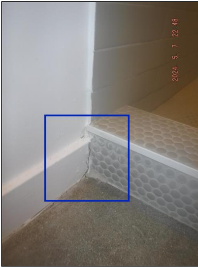
5.1 Item 1(Picture) Signs of water damage on wall
