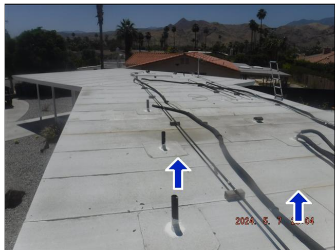
9.0 Item 2(Picture) Seem sealant failing
