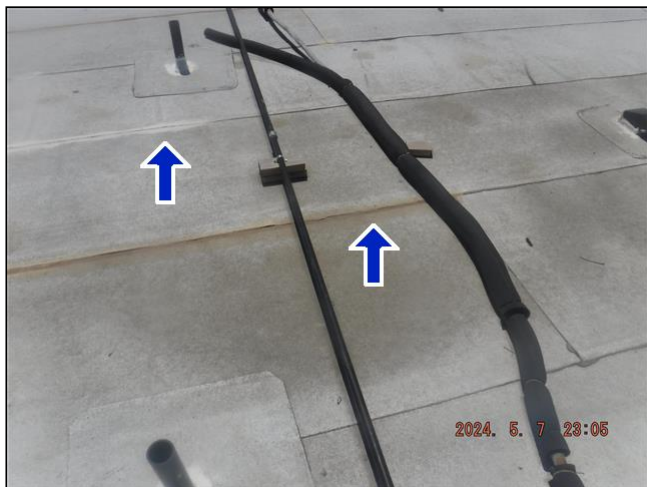
9.0 Item 3(Picture) Seem sealant failing
