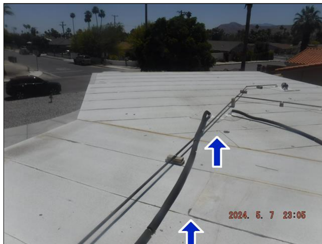
9.0 Item 4(Picture) Seem sealant failing
