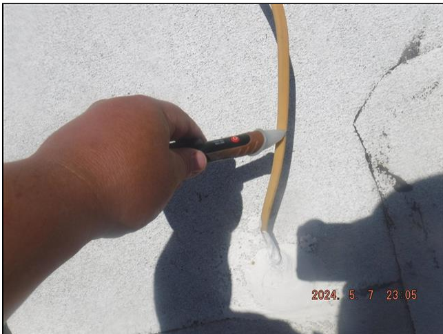
2.6 Item 3(Picture) Exposed electrical wiring (roof)
