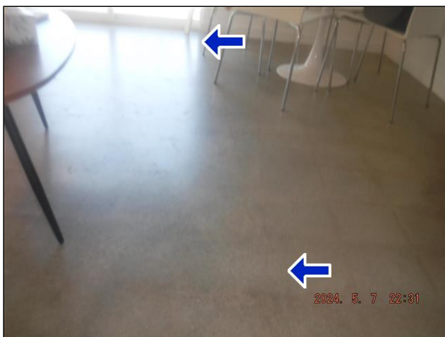
7.0 Item 1(Picture) Slab crack (living room)
