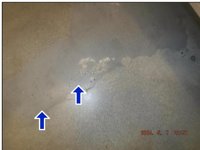
7.0 Item 3(Picture) Slab crack (master bath)
