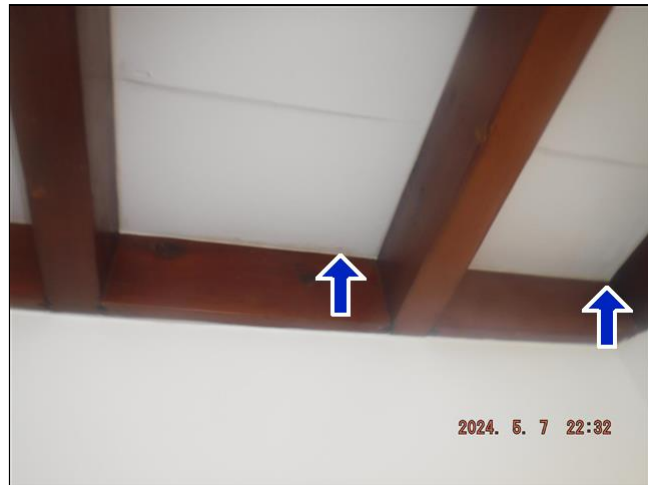
5.0 Item 4(Picture) Ceiling stains
