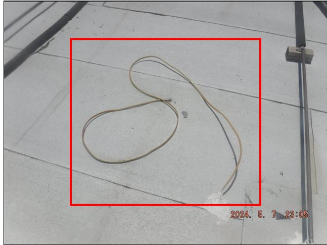
2.6 Item 2(Picture) Exposed electrical wiring (roof)
