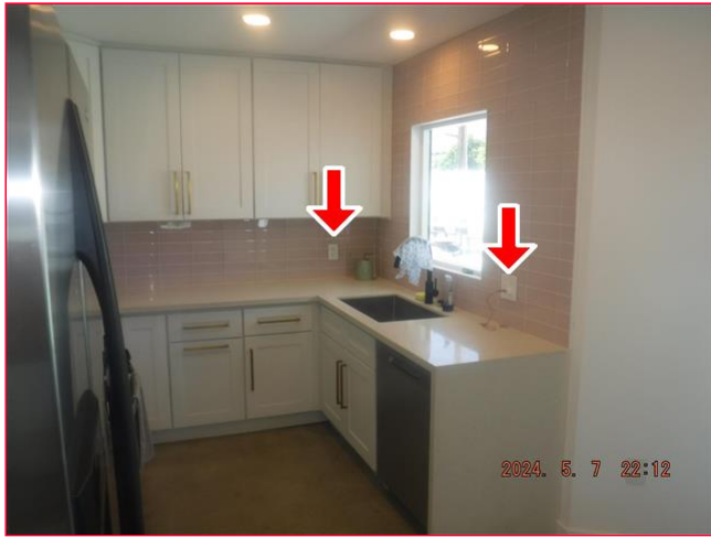
2.5 Item 1(Picture) No GFCI electrical outlet
