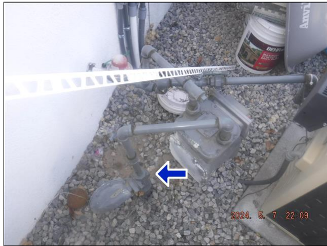
3.8 Item 2(Picture) Main Gas Shut Off (At Meter)
