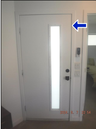
5.4 Item 1(Picture) Main entry door
