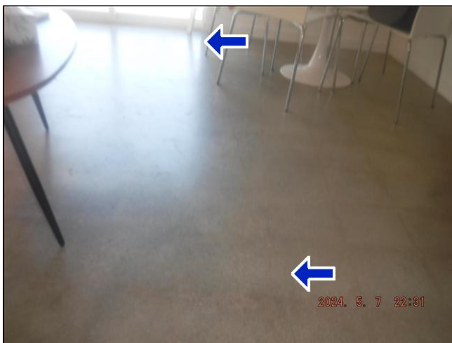
7.0 Item 1(Picture) Slab crack (living room)
