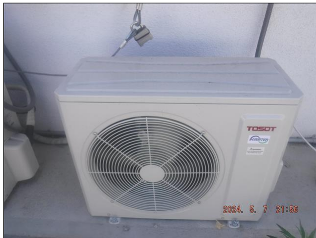
4.0 Item 2(Picture) Mini air conditioning unit 2
