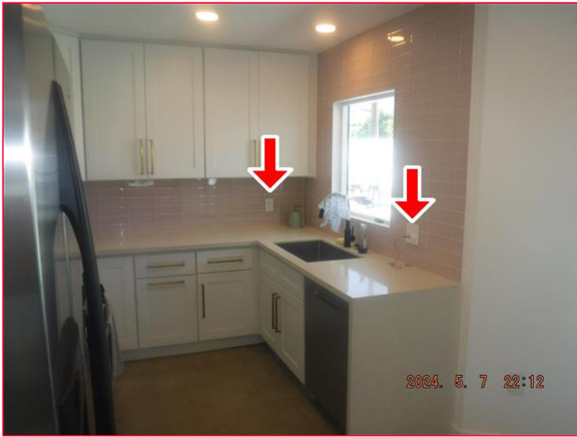
2.5 Item 1(Picture) No GFCI electrical outlet
