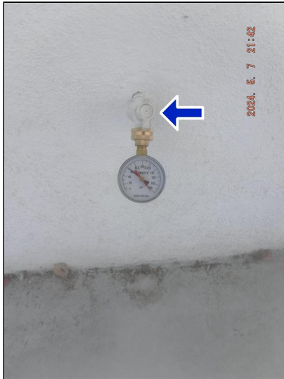
3.3 Item 1(Picture) Hose bib/ spigot (front of home)
