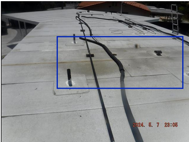
9.0 Item 5(Picture) Water ponding signs on roof
