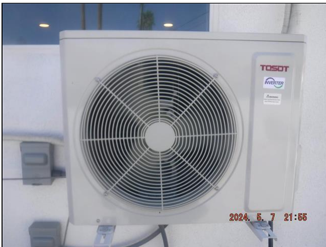
4.0 Item 1(Picture) Mini air conditioning unit
