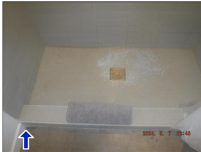
5.1 Item 2(Picture) Signs of water damage on wall
