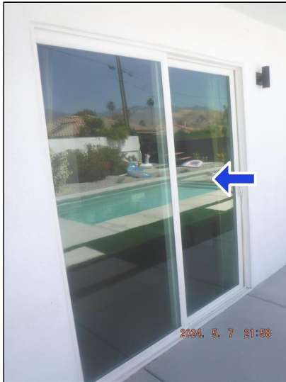
1.1 Item 1(Picture) Screen door missing
