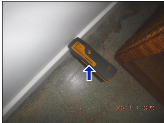
5.2 Item 6(Picture) Moisture meter (device) indicated dry surface
