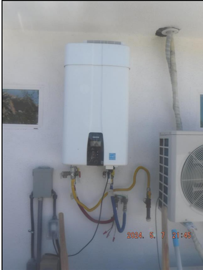
3.6 Item 1(Picture) Water Heater Unit
