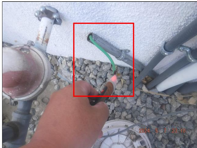
2.6 Item 4(Picture) Grounding wire at right side of home
