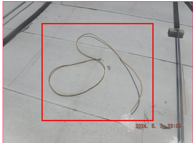
2.6 Item 2(Picture) Exposed electrical wiring (roof)
