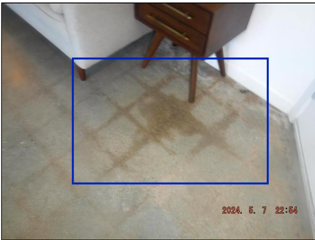
5.2 Item 5(Picture) Stained slab floor (living room)
