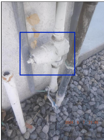
3.5 Item 1(Picture) Water pressure regulator location
