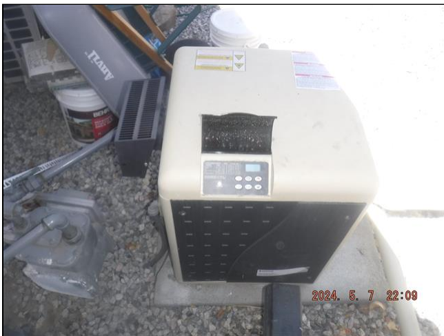
10.8 Item 1(Picture) Pool heating unit
