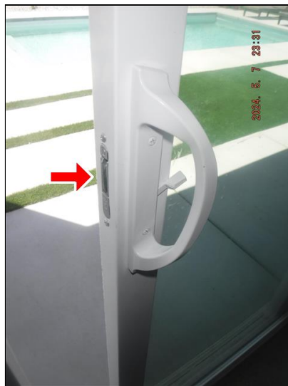
5.4 Item 4(Picture) Door did not lock properly
