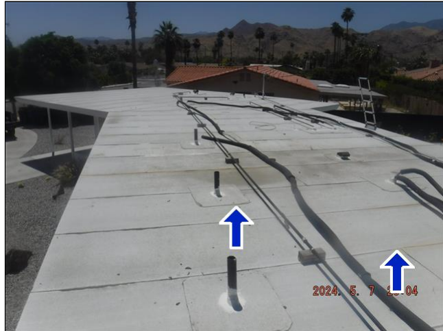
9.0 Item 2(Picture) Seem sealant failing
