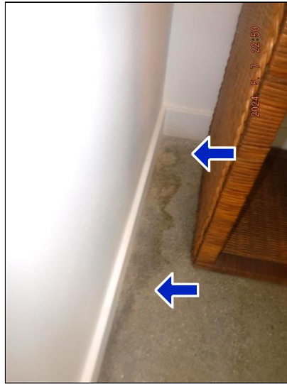
5.2 Item 4(Picture) Stained slab floor (master bedroom)
