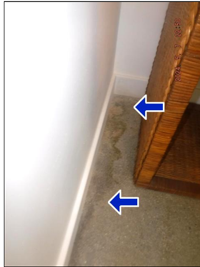
5.2 Item 4(Picture) Stained slab floor (master bedroom)
