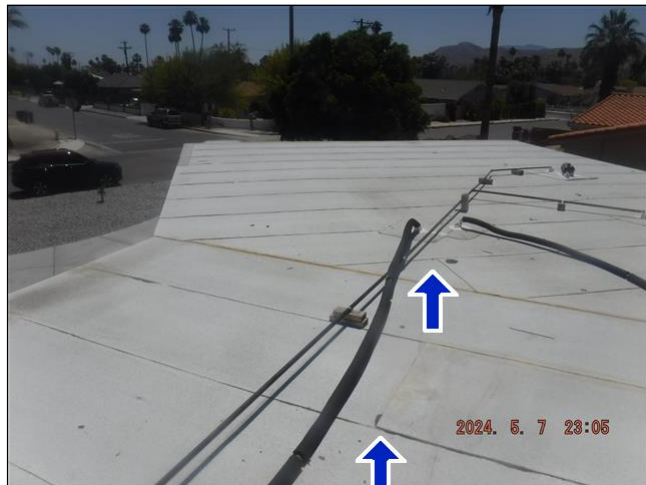
9.0 Item 4(Picture) Seem sealant failing
