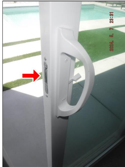
5.4 Item 4(Picture) Door did not lock properly
