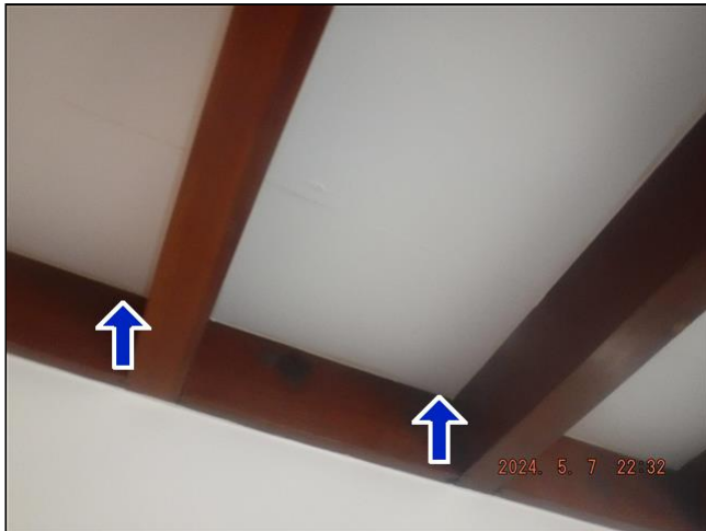
5.0 Item 3(Picture) Ceiling stains
