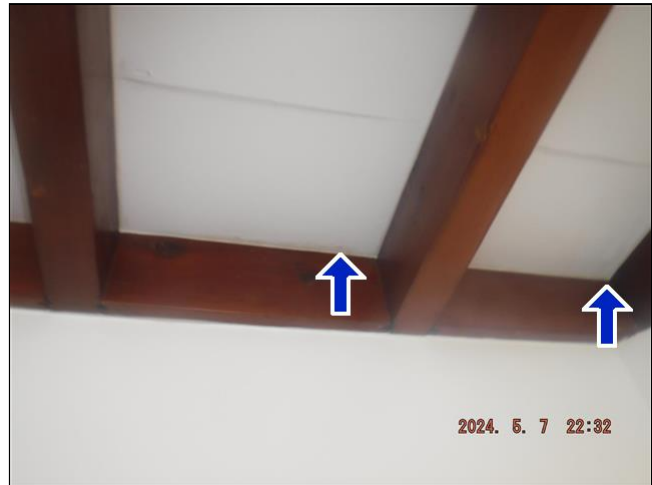
5.0 Item 4(Picture) Ceiling stains
