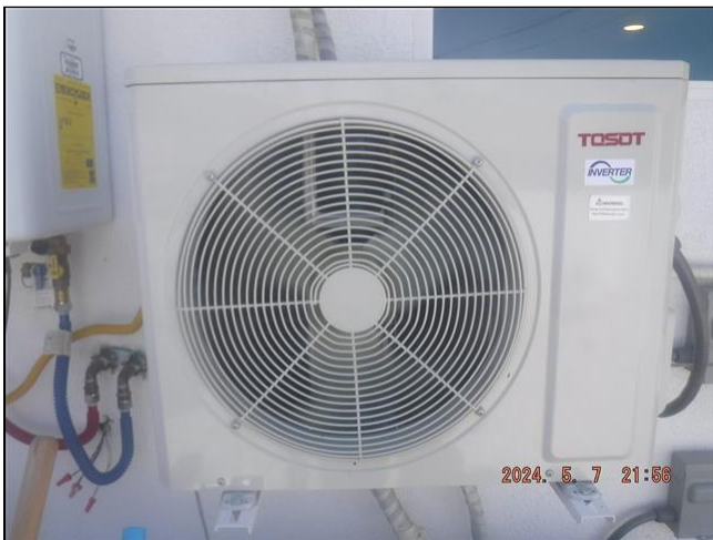
4.0 Item 3(Picture) Mini air conditioning unit 3
