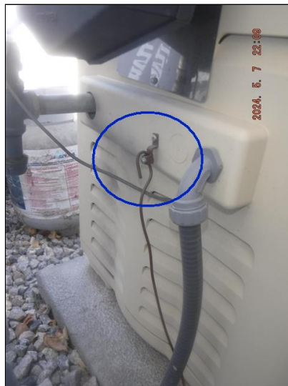
10.8 Item 2(Picture) Heating unit bonded/grounded for safety
