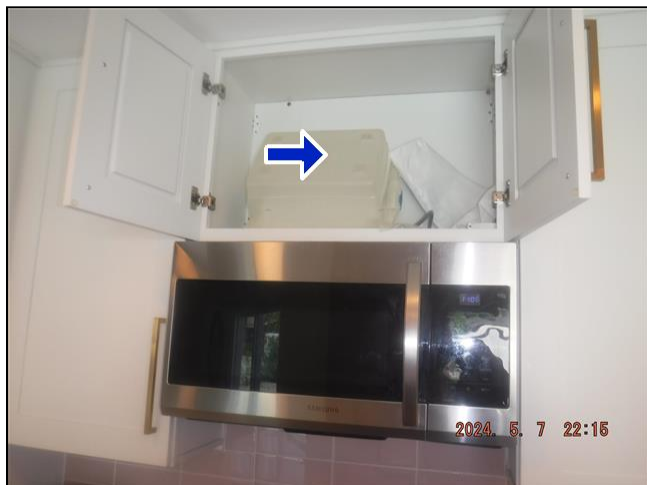
6.4 Item 1(Picture) Range hood fan not vent outdoors
