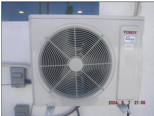
4.0 Item 1(Picture) Mini air conditioning unit
