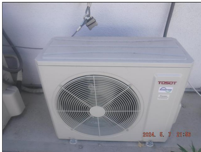
4.0 Item 2(Picture) Mini air conditioning unit 2
