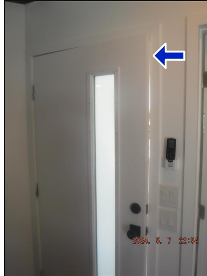
5.4 Item 2(Picture) Door rubs at top
