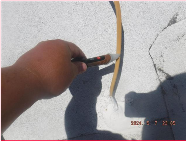
2.6 Item 3(Picture) Exposed electrical wiring (roof)
