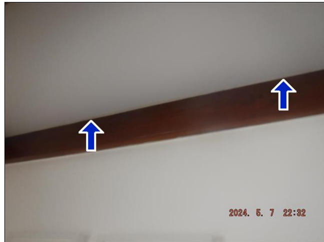
5.0 Item 2(Picture) Ceiling stains
