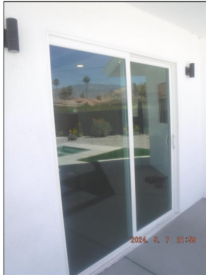
1.1 Item 2(Picture) Screen door missing
