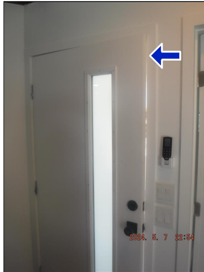
5.4 Item 2(Picture) Door rubs at top
