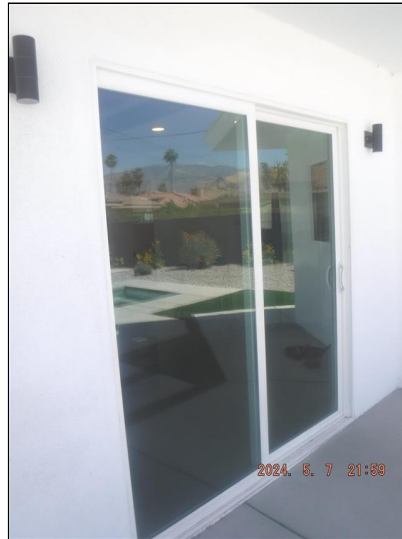
1.1 Item 2(Picture) Screen door missing
