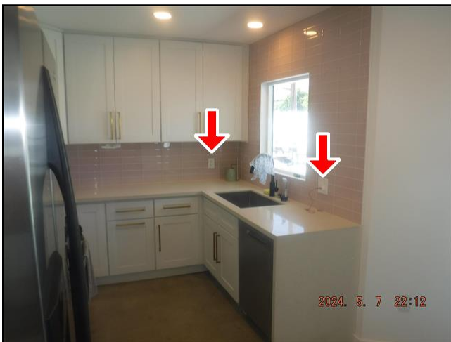
2.5 Item 1(Picture) No GFCI electrical outlet
